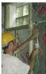
Above left/right Triple-glazed windows, super-insulation and airtight details eliminate draughts and condensation, and ensure low levels of heat loss; super-insulation standards can be achieved without affecting the external appearance. Below Teaching the skills of airtight construction will be crucial in the retrofit roll-out.
