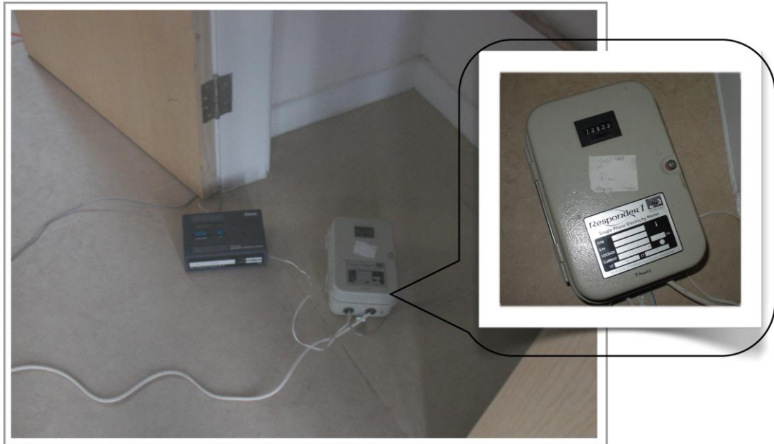
Figure 2.4 Pulse KWh electricity meter and data logger
