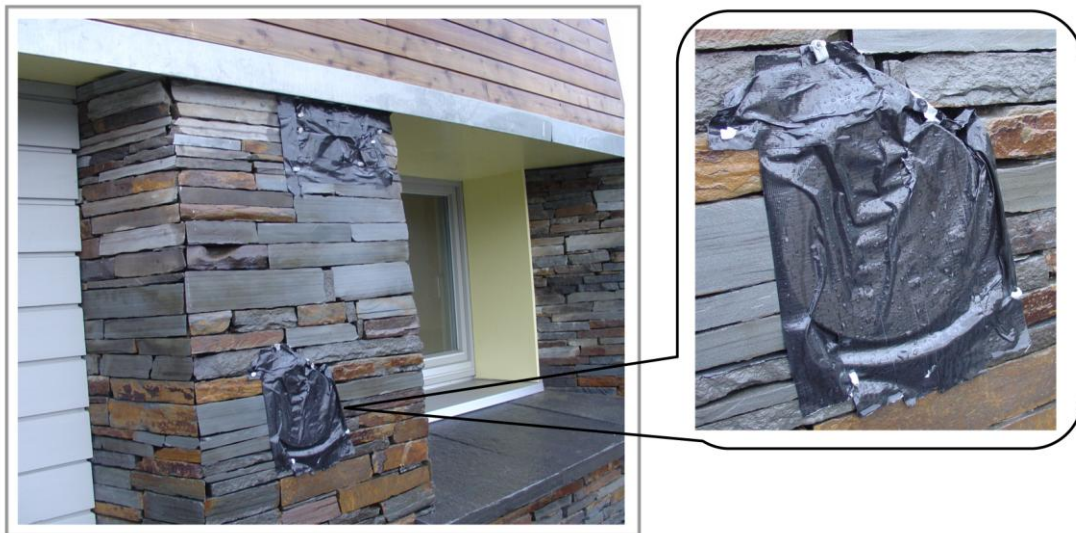
Figure 2.1 Sealed MVHR inlet & outlet (the Larch House)
