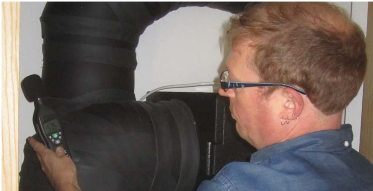
Green Building Store's Andrew Farr re-balanced the HRV after airtightness and other system tests
