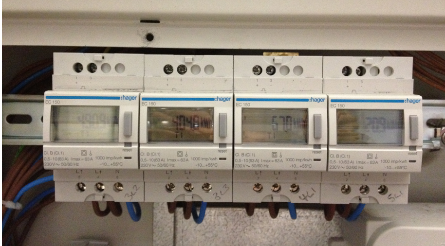
Mayville Community Centre - sub-meters
